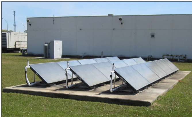
A solar water heater outside B-1104 is used to lower energy costs associated with domestic heating.
