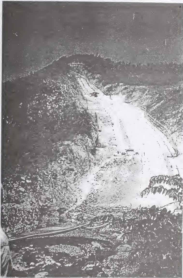
Figure 5: West side of Portugues Dam site. Grout pipes are visible to right of rails.
