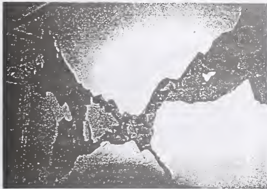
Photo 13 Damage of brick wall of the high-rise residential building (Fengyuan City, Taichung County)
