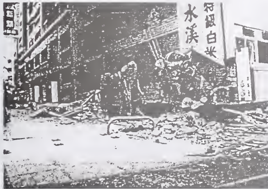
Photo 15 High-rise multiple dwelling house in which first floor collapsed (Taichung City) Destruction situation of the first floor column in photo 14. The damage of the lower part is being concentrated at first floor.
