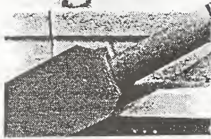
Wind Damage - Fractured Guide Pipe
