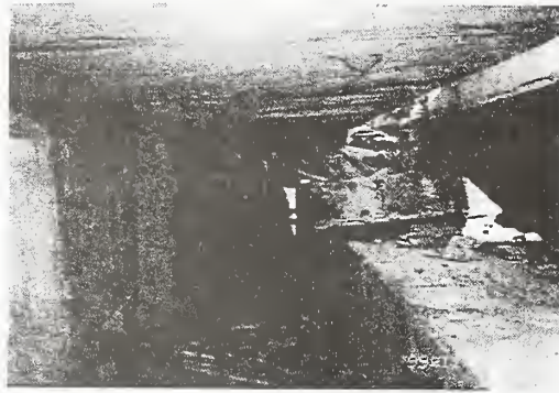
Photo 11 Damage at Expansion Joint and Bearings (Courtesy of H. Hoashi)
