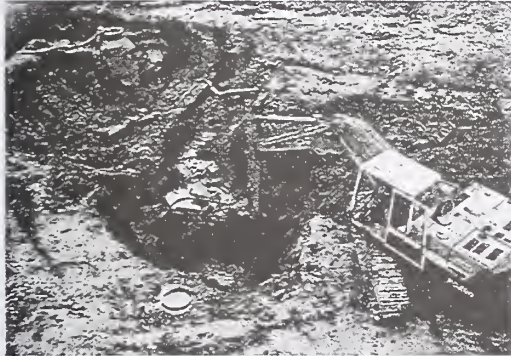
Photo 3 Offset of a Sewage Pipe (Point H, refer to Fig. 3)
