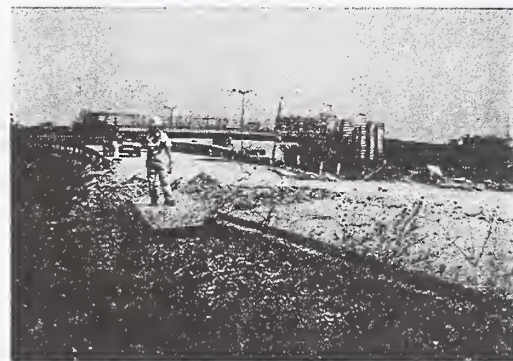
Photo 7 Minor Damage in an Overpass where the Fault Crossed the Overpass at Its Abutment
