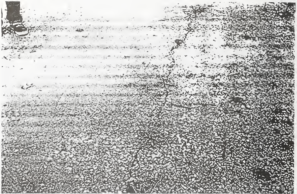
Figure 3. Longitudinal crack near the edge of the crest of Gokce Dam on the upstream side. The location is about at the middle of the dam. The width of the crack was about 7 mm at its greatest
