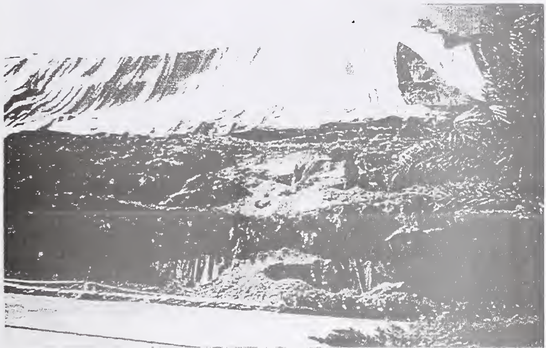
Photo.2 Front view of the collapsed geosynthetic-reinforced soil retaining wall(Site2 in fig.1)
