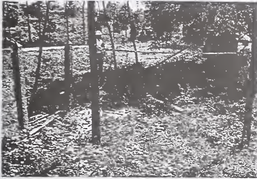
Photo 1 Offset of a Concrete Fence of 4.3 m at Automobile Factory (Point D, refer to Fig. 3)
