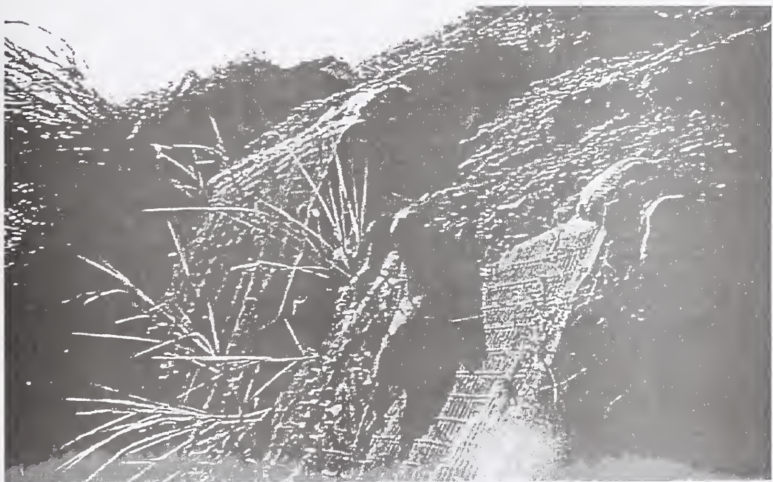
Photo.3 Failure of the reinforcement
