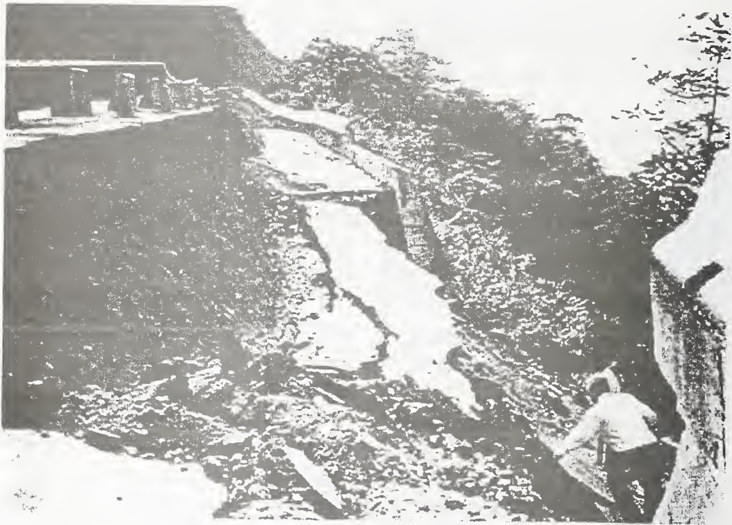
Photo.1 Collapsed gravity-type concrete retaining wall (Site1 in Fig.1)
