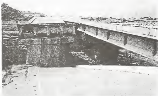
Photo 13 Collapse of Wu-Shi Bridge
