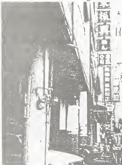
Photo 11 Damage of the column in the first floor setback division (Tungshih, Taichung County)
