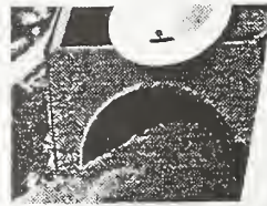
Wind Damage - Fractured Guide Pipe
