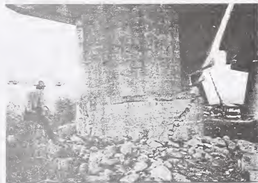
Photo 14 Failure of Caisson Foundation as a Direct Fault Movement, Wu-Shi Bridge (Courtesy of S. Iwata)
