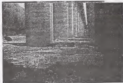
Photo 10 Fault that Crossed 10-Span Bridge (Courtesy of H.Hoashi)
