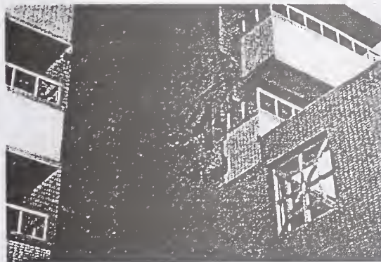
Photo 17 Damage of the middle floor of the high-rise multiple dwelling house (Fengyuan City, Taichung County)
