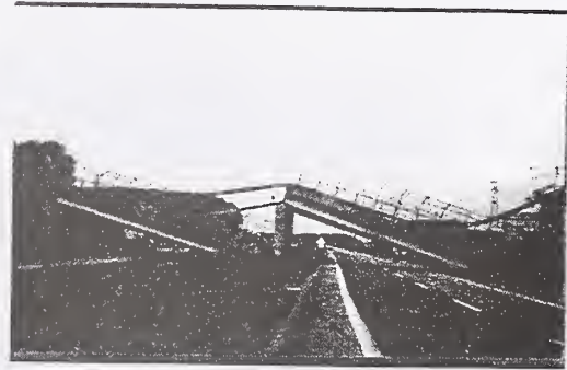
Photo 6 Collapse of Arifiye Bridge (Courtesy of H. Hoashi)
