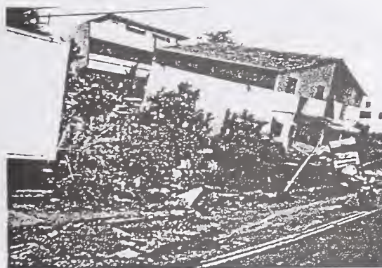
Photo 5 Building just above fault (Fengyuan City, Taichung County) The ground behind building is rised. The building in this vicinity got same damage
