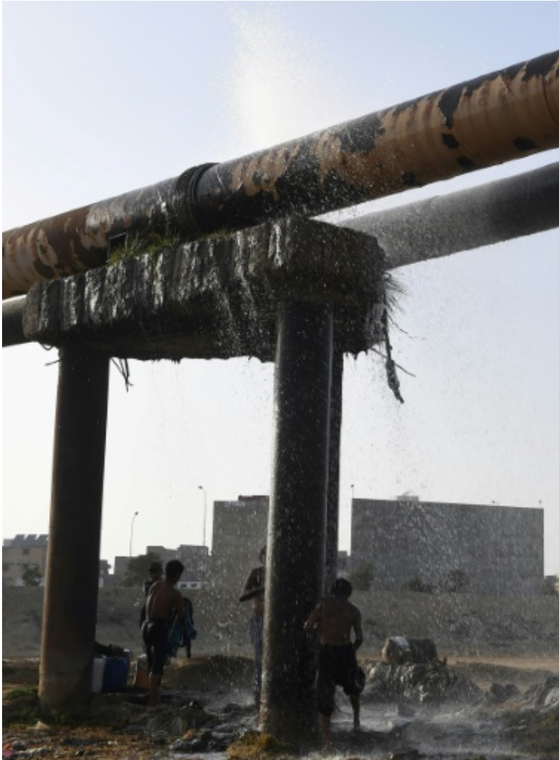
Karachi youngsters cool off under a leaking water pipeline
